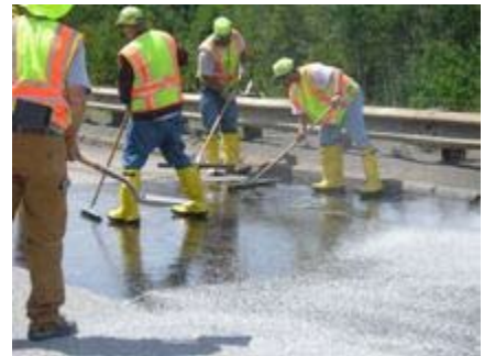
A thin layer of 3/8-inch-minus aggregate is spread over the epoxy. Loose aggregate is later swept from the surface.
