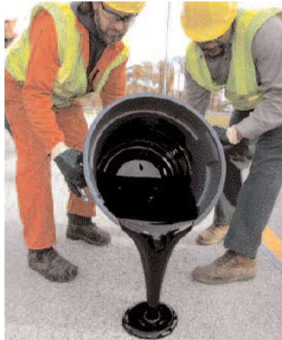
Safelane is a patented combination of epoxy and aggregate rock, which can be installed in the summer
