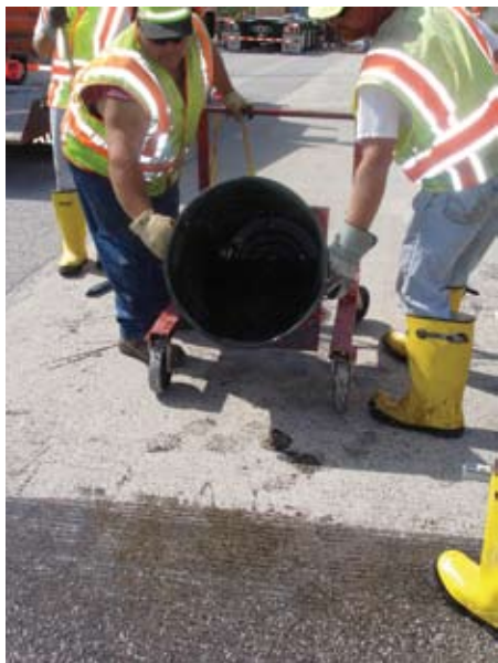
Fig. 1: After surface preparation, an initial 1/8 in. (3 mm) thick layer of epoxy is applied to the bridge deck
