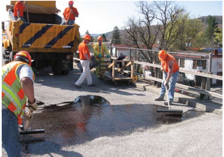
Fig. 3: After the first layer cures, a second layer of epoxy and aggregate is applied to a total thickness of 3/8 in. (10 mm)
